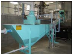
Influent screens (top) Vortex grit system
